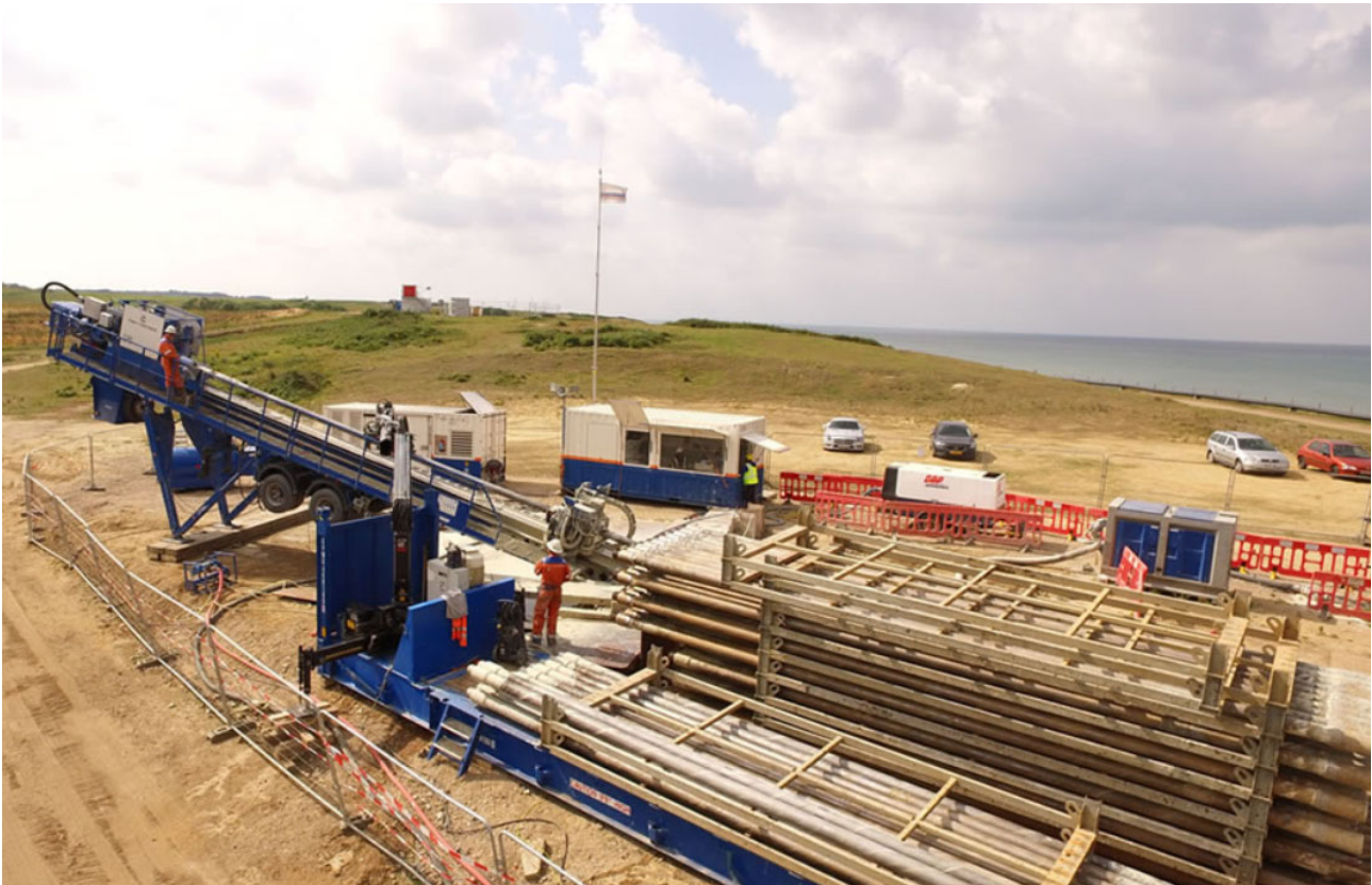
Plate 4-12: Example of an onshore landfall compound (DOW) with drilling rig (left of shot) in operation (Source: Equinor)
